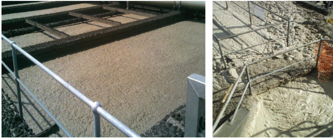
Figure 1. Foam covering the surface of an aeration basin and walkways.
